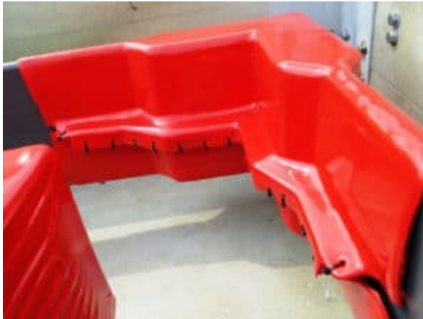
Figure 3: New style insulating boots with tie-wraps on side
