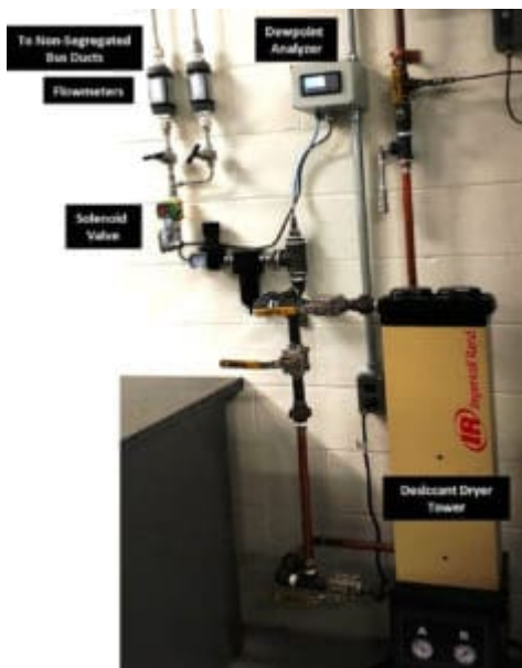
Figure 6: Dry air injection and protection equipment
